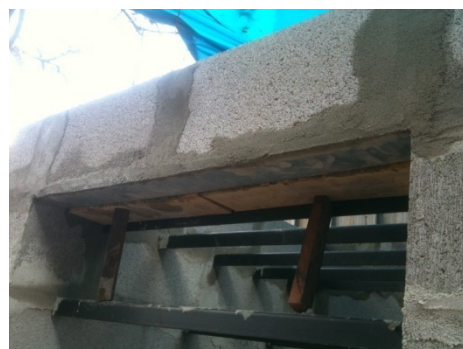
14. Timber formwork pieces supported under front besser bricks to hold concrete in place.
