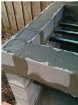
13. Fill besser brick holes with scraps of brick and concrete, stuff with paper, fill top with concrete. (see #11 – could fill them with concrete from the bottom and reinforce...)
